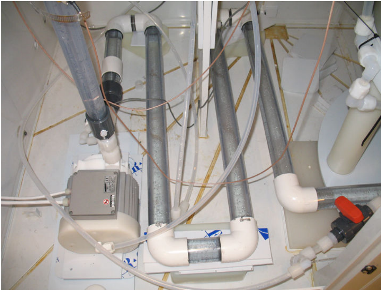
Figure 8. Collection of gas in the supply line after prolonged shutdown
